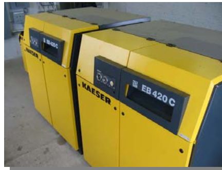
The installation conducted by Hope Air Systems at NH Gas, included two Kaeser Model EB 420C 50 HP blower units and two Kaeser Model BB 88C 10 HP blower units integrated with a pressure and flow controller package designed by Sorensen Systems.
