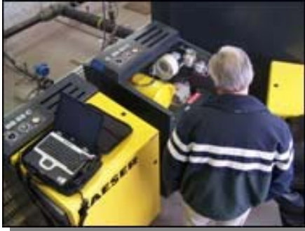
Marc LeBaron, Project Manager for Sorensen Systems, inspects one of the four Kaeser Omega Blowers installed as part of the propane gas control system developed for NH Gas in Keene, NH.
