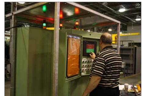
The electronic control enclosure, which was programmed by The Hope Group engineers, is equipped with a stack-light assembly consisting of green, amber and red indicator lights, with each light indicative of the overall status of the three pump stations.
