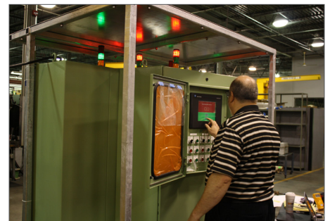
The electronic control enclosure, which was programmed by The Hope Group engineers, is equipped with a stack-light assembly consisting of green, amber and red indicator lights, with each light indicative of the overall status of the three pump stations.
