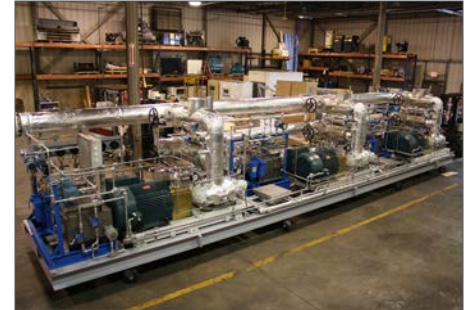
The compact design of the skid accommodated three pump/motor combinations working in parallel, each pump drawing oil from a common supply and discharge header and each pump/motor has its own electrical controls and protective devices
