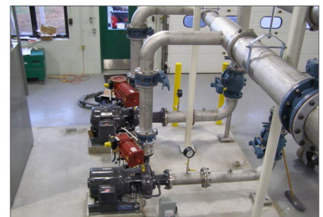
According to officials from the Keene, NH, Public Works Department, this is the first installation of this kind in New Hampshire and represents an opportunity for gravity-fed water system deploying regulator valves.
