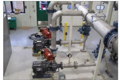
According to officials from the Keene, NH, Public Works Department, this is the first installation of this kind in New Hampshire and represents an opportunity for gravity-fed water system deploying regulator valves.
