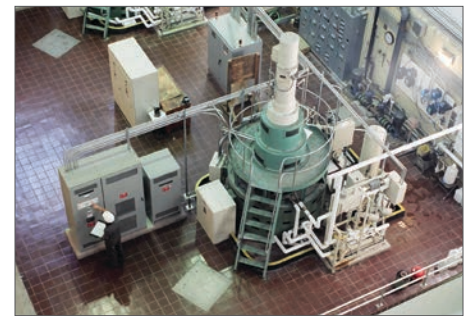
Sorensen Systems upgraded and refurbished the two 1.6 MW generators at the MWRA Cosgrove Intake facility in Massachusetts.
