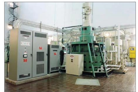
Sorensen Systems built two new digital excitation control systems as part of refurbishment.
