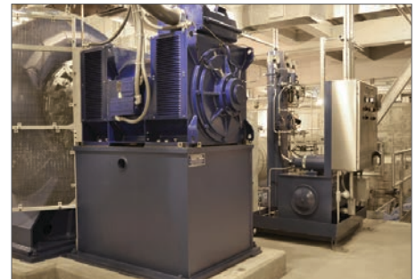
The 200 kW, 480 VAC, 3PH, 60 Hz, 727 rpm induction generator was manufactured by Marelli Motori.
