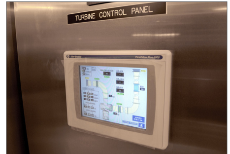
The custom built Turbine Control Panel used Allen-Bradley SLC500 PLC and Panelview Plus HMI.
