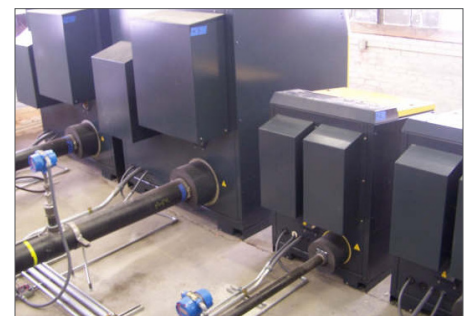
The ambient air, gravity-fed system needed a boost from the low-pressure blowers as demand for propane gas increased from residential and commercial expansion.
