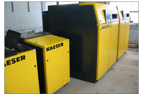
The four low pressure blowers installed at NH Gas in Keene NH were designed to cover a wide cfm range and to serve as internal back-up during routine maintenance.
