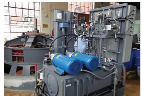
The Spartanburg Water Treatment plant operates two 500 kW turbine generators providing water treatment and power generation to 200,000 consumers including neighboring counties.
