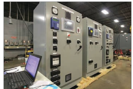
The refurbishment included new PLC based unit control systems, one per generator, which were programmed and tested at the Sorensen Systems fabrication facility.
