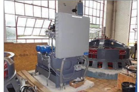
Sorensen Systems designed and built turbine control panels and balance of plant control panels as part of the Spartanburg Water Treatment improvement project.
