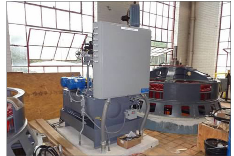
The Hope Group designed and built turbine control panels and balance of plant control panels as part of the Spartanburg Water Treatment improvement project.
