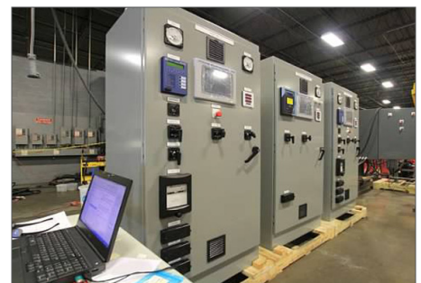
The refurbishment included new PLC based unit control systems, one per generator, which were programmed and tested at the The Hope Group fabrication facility.
