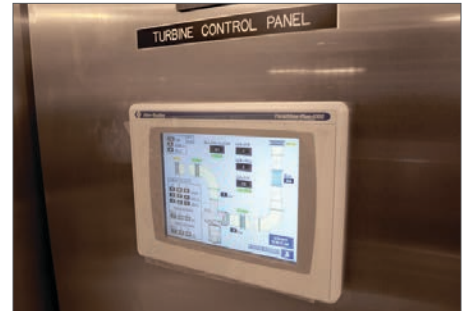
The custom built Turbine Control Panel used Allen-Bradley SLC500 PLC and Panelview Plus HMI.
